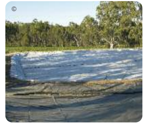
VapourGuard™ cover installed by Fabtech
